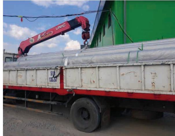
Vinhomes Grand Park project – district 9 – Ho Chi Minh City
